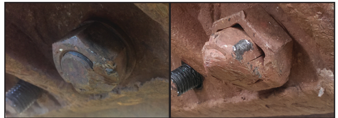
FASTENER ABRASION AND WEAR
